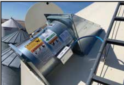
Roof exhaust fans to assist in reducing condensation when in-bin drying
